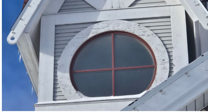
Photo showing signs of paint flake and weathering.
