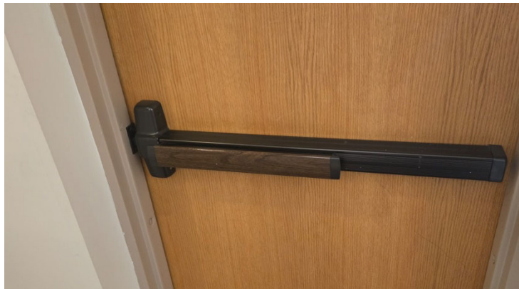
Photo showing panic device hardware at egress point.
