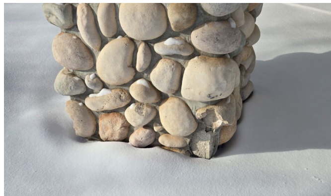
Photo showing stone veneer damage.
