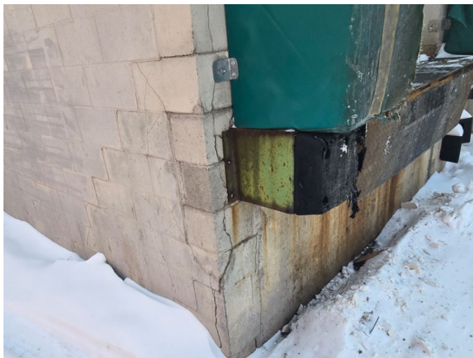
Deterioration at loading dock leveler.
