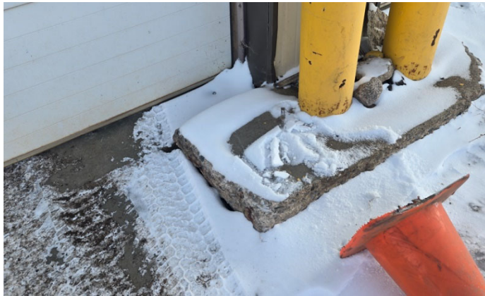
Photo showing one of the raised bollard piers infringing on overhead door entry.
