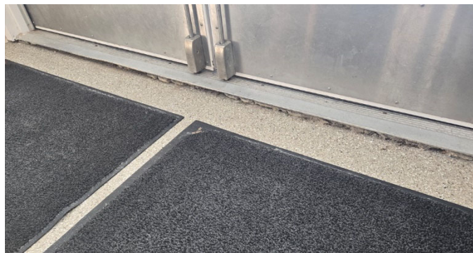
Photo showing raised sill/trip hazard at east entrance.
