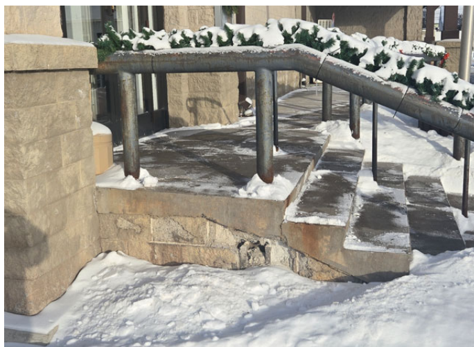
Deterioration at entry steps and guardrail.
