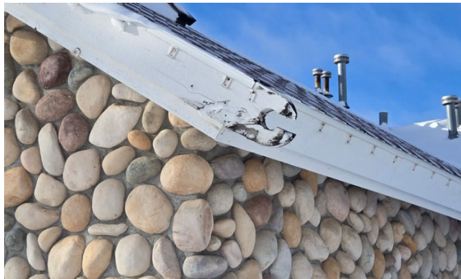
Photo showing wood decay at decorative element.
